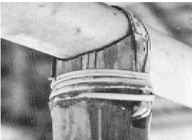
fig 7.3 Illustrates how the top rung of the structure will be secured. The uprights will be cut into a U-shaped cup that is approximate to the size of the culm that will sit within it. The posted upright is drilled with a 1/2 inch drill bit 3 inches below the highest point of the upright. Green bamboo lashing will be used to lash the connection together.
