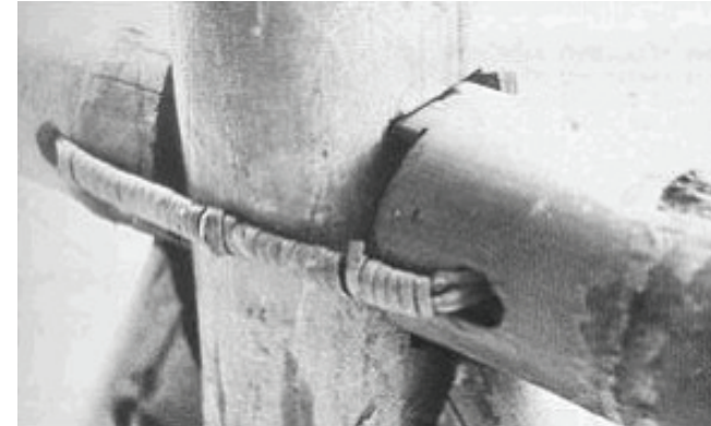
fig. 7.2 The horizontal culms drilled and tied similarly to figure 7.3; the interlocking key of this makes the vertical connection secure.
