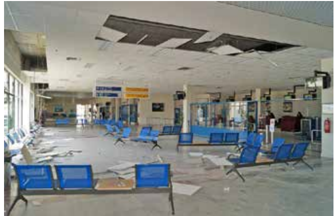
Figure 37. In 2014, a M6.9 earthquake near Greece caused nonstructural damage to airport at Lemnos International Airport in Lemnos, Greece. Photo: Ayis Theos.
