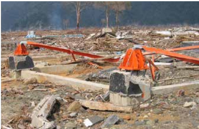
Figure 106. The 2004 Indian Ocean tsunami compounded communication infrastructure damage already caused by the earthquake, including completely knocking over cell towers. Widespread damage to communication systems can delay the response time of emergency services and leave survivors without crucial information. Source: USGS.
