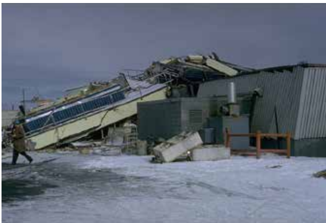
Figure 36. The Great Alaskan Earthquake in 1964 caused this reinforced concrete-framed control tower to collapse at the Anchorage International Airport. Photo: Karl V. Steinbrugge.
