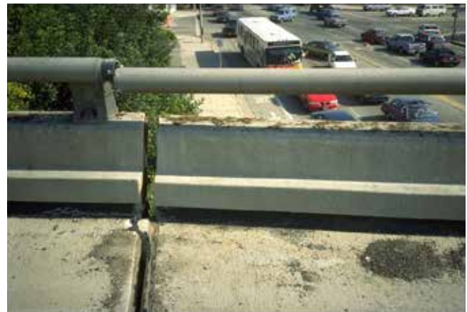
Figure 25. The 1994 M6.7 Northridge Earthquake caused low damage to a California highway bridge, shifting sections of the bridge and breaking a guard rail. Bridges with low damage should be operational and require only minor repair later. Photo: Mark Aschheim.
