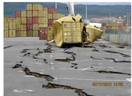
Figure 7. Damage due to liquefaction and lateral spreading at the Port of Coronel in Chile after the M8.8 Maule earthquake. Port facilities are particularly vulnerable to damage from lateral spreading. Photo: Geotechnical Extreme Events Reconnaissance (GEER).
