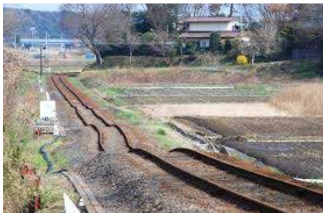
Figure 43. The 2011 M 9 Tohoku earthquake caused considerable bending of the Hitachinaka Railway tracks. Photo: Toshinoei Baba.
