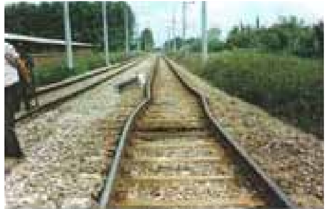
Figure 42. The M 7.4 earthquake in Turkey caused localized bending of the rail tracks. Photo: Turkish State Railways.
