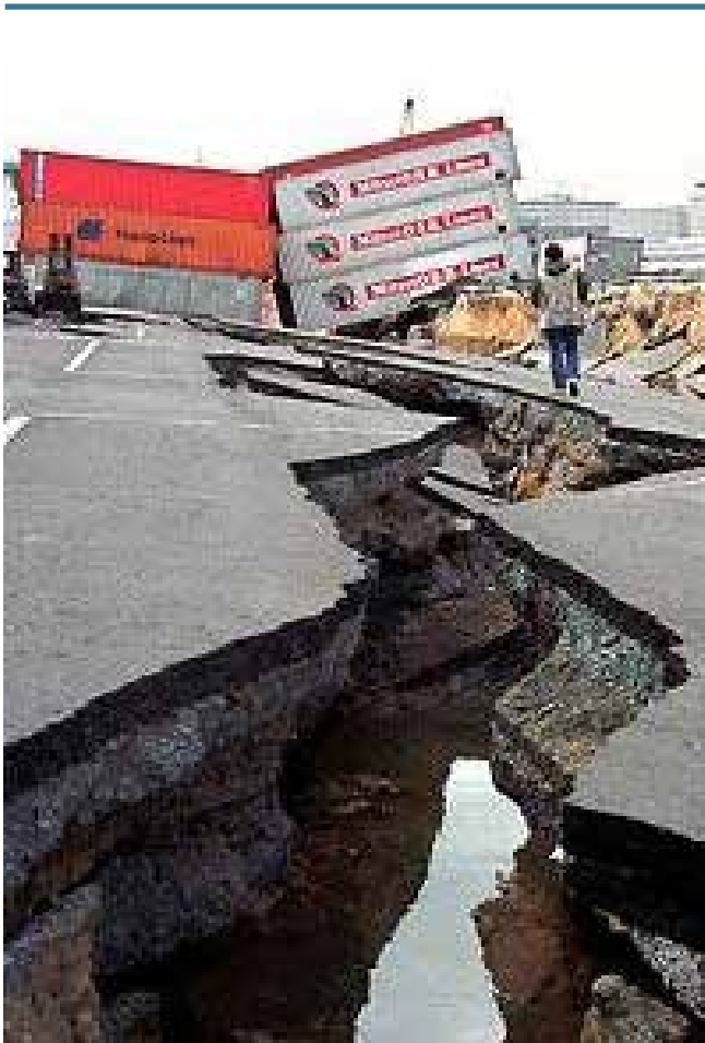
Figure 47. Liquefaction resulting from 1995 M 6.9 Kobe earthquake caused high damage to facilities at the Port of Kobe. The liquefied soil pushed against a major retaining wall causing it to slide five to ten feet toward the water. This movement caused settlement of the retained soils and destroyed structures supported by these soils. Photo: Koji Sasahara, AP.
