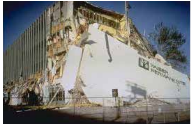
Figure 80. In the 1994 Northridge earthquake high damage to hospitals and medical facilities limited medical response to injured survivors and patients with on-going medical needs. Photo: M. Celebi, USGS.
