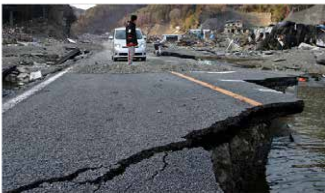
Figure 17. The 2011 Tohoku tsunami caused high damage to roadways, shifting parts of the road up or down by more than a foot. Photo: Japan Red Cross Society, published in the New York Times March 24, 2011.
