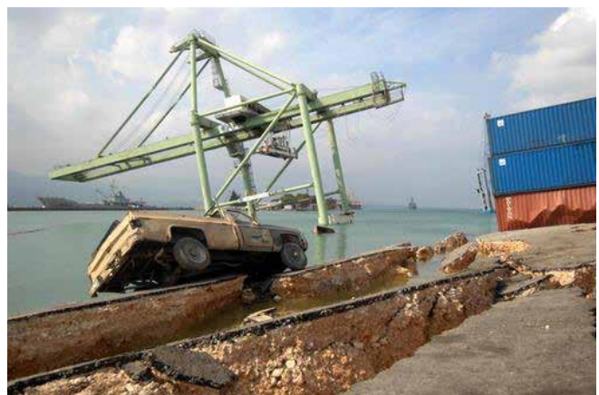
Figure 49. The 2010 M7 Haitian earthquake caused high damage to the main port terminal in Port-au-Prince. Seismically induced lateral spreading caused a shipping-container crane to tilt toward the harbor. Photo: Daniel C. Pearson, U.S. Navy.
