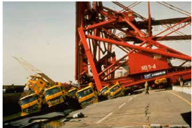
Figure 53. The 1995 M6.6 Kobe earthquake damaged a loading ramp structure at Higashi-Kobe ferry pier, along with other port infrastructure in the area. Damage to ferry facilities could isolate island populations in the San Juan Islands and slow transportation across the Puget Sound. Photo: unknown.
