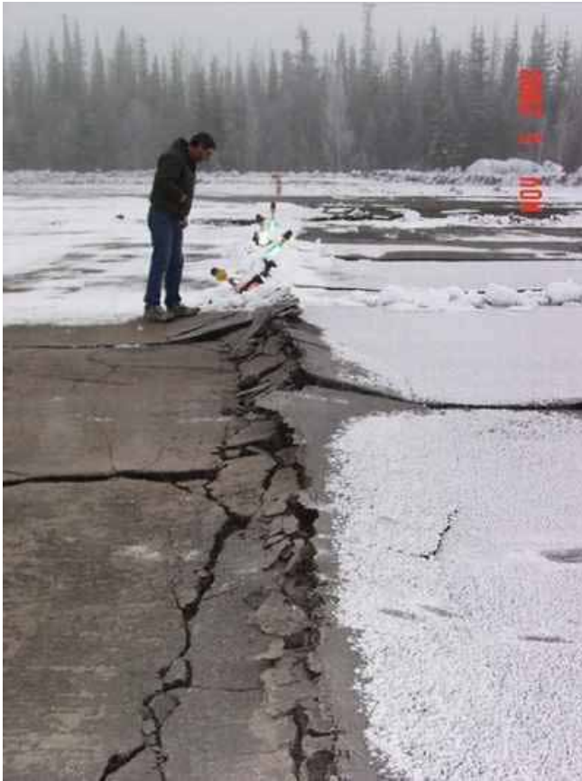
Figure 38. The M7.9 Denali earthquake in 2002 caused significant damage to the only runway at the Northway, Alaska airport. The runway was temporarily replaced with a gravel surface before permanent repairs. Photo: Unknown.
