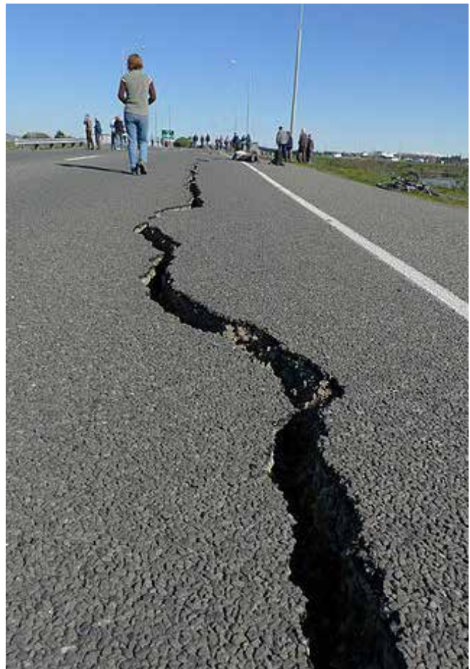
Figure 18. The 2010 M7.1 Canterbury, New Zealand earthquake caused low to medium damage to roadways, with two to five inches of permanent ground displacement. Photo: Martin Luff.
