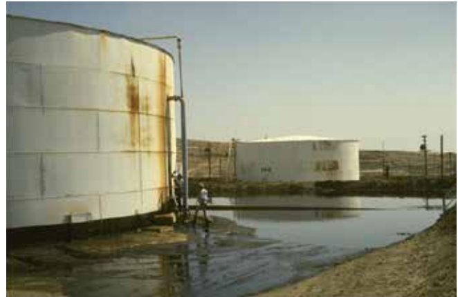
Figure 100. Shaking from the 1983 M6.5 Coalinga earthquake caused the pipe connections to break at a Chevron facility. Oil spilled out of the damaged connection, but was retained by dikes. Photo: Karl V. Steinbrugge.
