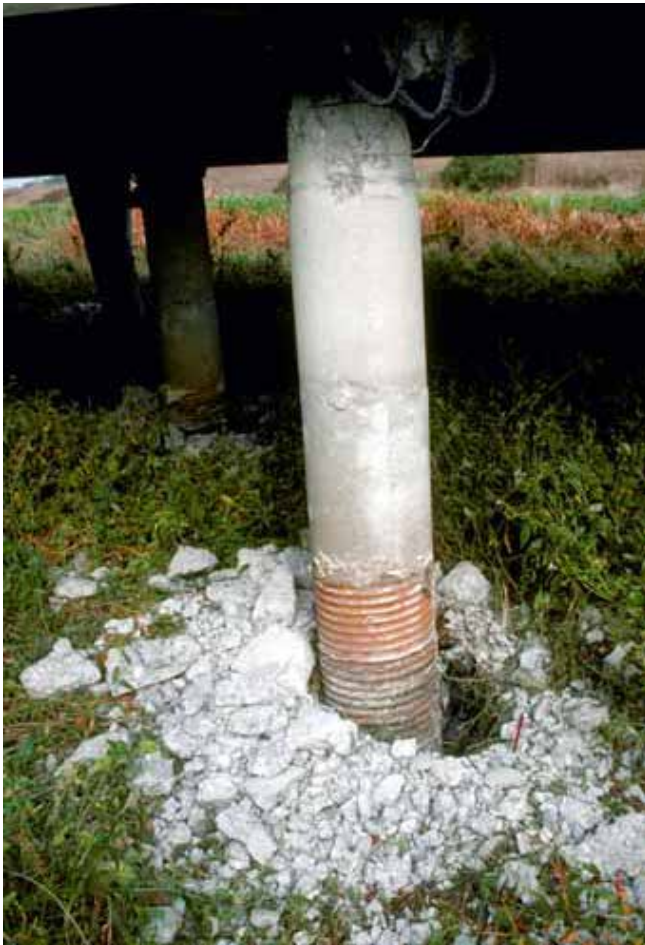
Figure 24. The 1989 M6.9 Loma Prieta earthquake in California caused medium damage to the support column of a bridge. The shaking caused the concrete to break up and shift the bridge column alignment. Photo: H.G. Wilshire, USGS.
