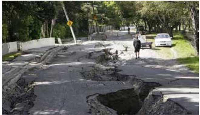
Figure 20. The 2011 M6.3 Christchurch, New Zealand earthquake caused high damage to roadways as a result of ground failure due to liquefaction. This type of damage may require the removal and replacement of existing pavement. Photo: David Hallett, HITRAC.
