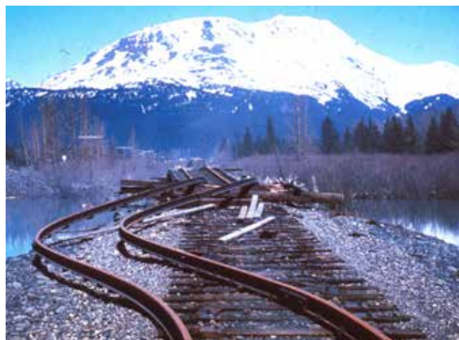
Figure 44. The M9.2 Great Alaska Earthquake of 1964 damaged extended lengths of track due to ground failure as a result of lateral displacement. This type of ground failure can tear rails from their ties and caused them to buckle. Photo: USGS.
