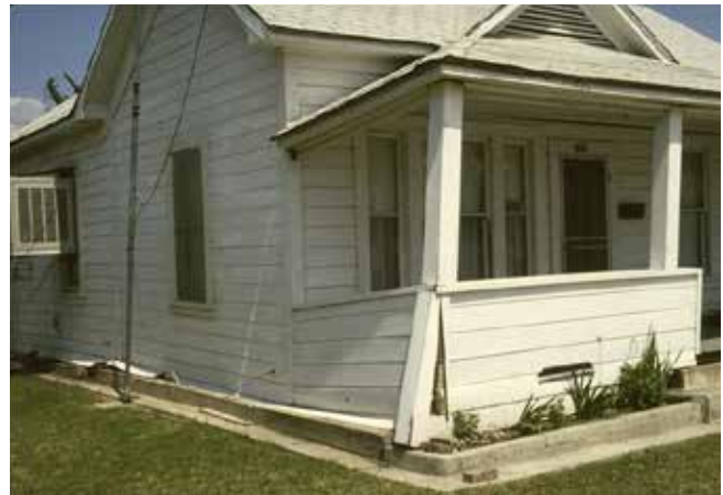
Figure 113. The 1983 M 6.2 Coalinga earthquake caused the cripple walls of wood-frame houses to fail, resulting in the house sliding off its foundation. Wood frame houses are flexible enough that collapse is unlikely for most of them, but many built prior to 1976 are at risk of shifting off of their foundations. Photo: Karl V. Steinbrugge.
