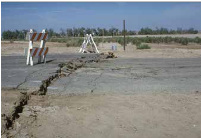
Figure 19. A M7.0 earthquake in California caused medium damage to roadways, with three to twelve inches of vertical displacement dissecting the road. This type of damage can be patched with an asphalt concrete overlay. Photo: Karl V. Steinbrugge, HITRAC.
